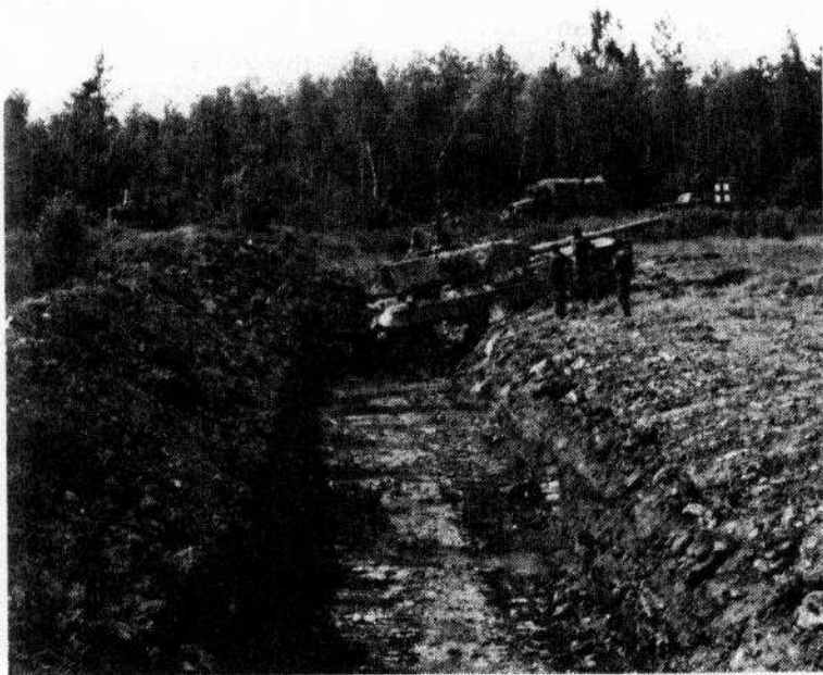
(Fig 1) The Leopard dozer quickly fills in and crosses a rectangular ditch.
